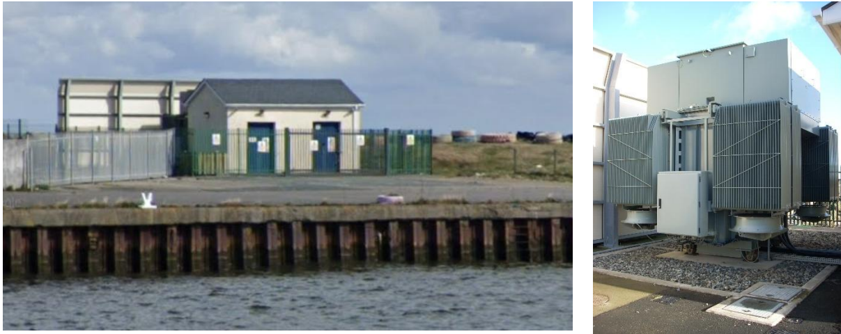
Plate 3.2: Fenced onshore substation compound within the Onshore Site observed from the west (left) and transformer (right)
